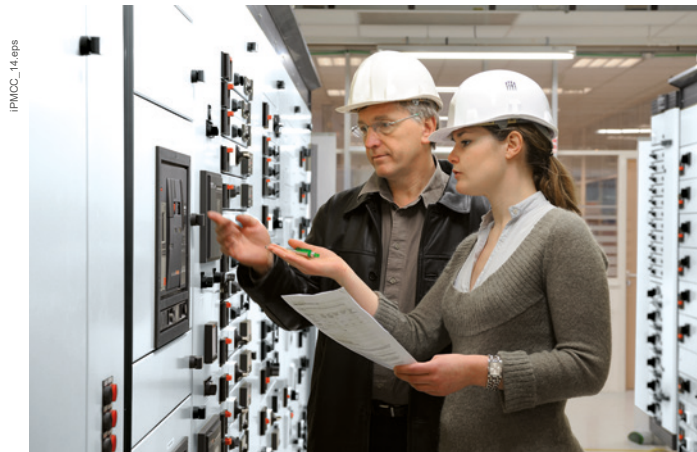
Motor Control Centre (MCC)
