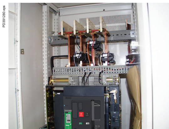
CT on vertical busbars.
