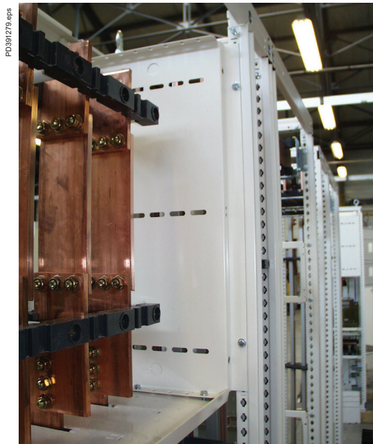
Dismountable vertical busbars.
